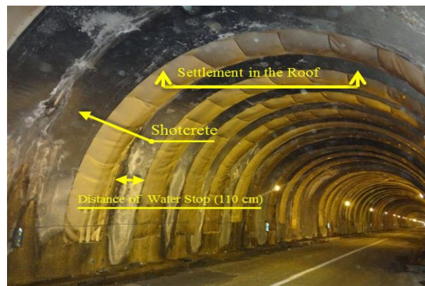
Fig. 4. Settlement in Tunnel Roof.
