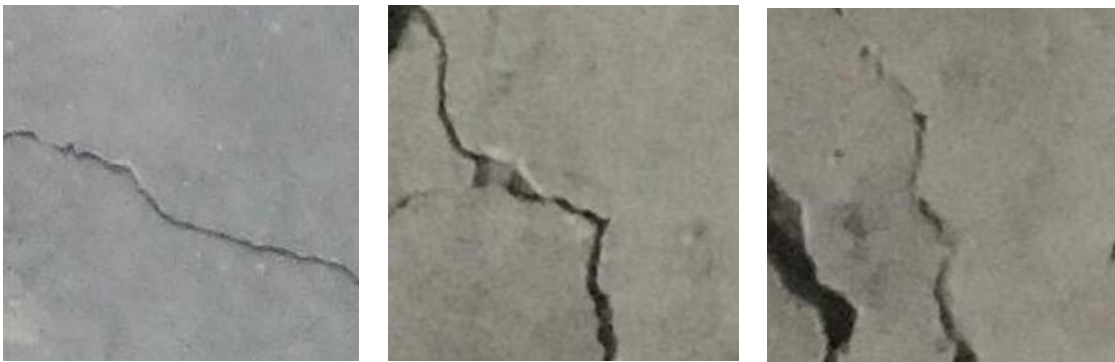
Fig. 1. Concrete surface with cracks (Sample from dataset used in this research).
