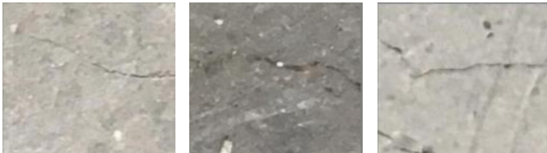
Fig. 6. Cracks not detected by model.
