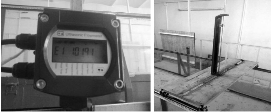
Fig. 1. Ultrasonic Flowmeter and Point Gage.
